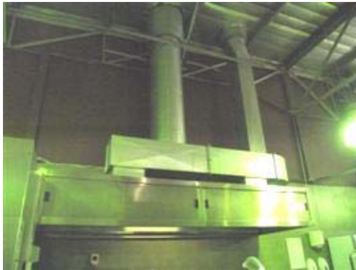
2 x Stainless Steel Fume Extraction Hood With Ducting Photo 49, 50
